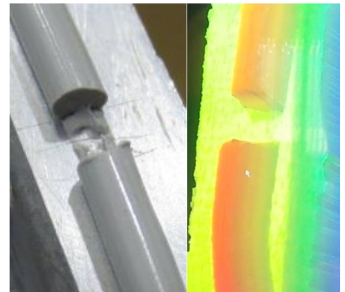
Missing a chunk of bead
